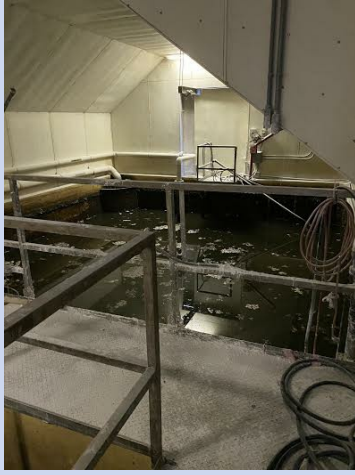
Water treatment process at Tehama. Photo by Lorin Letendre
